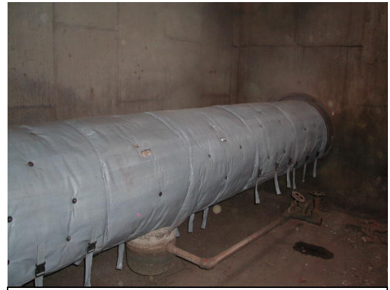
Double Slip Expansion joint & Piping
