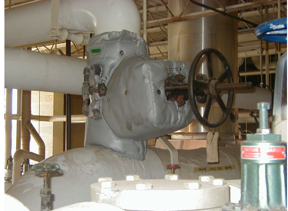
8” 250# Gate Valve – 150 psi Steam Header
