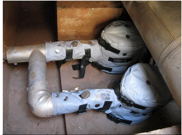
Spirax Sarco Condensate Pumps Manhole Steam Pit
