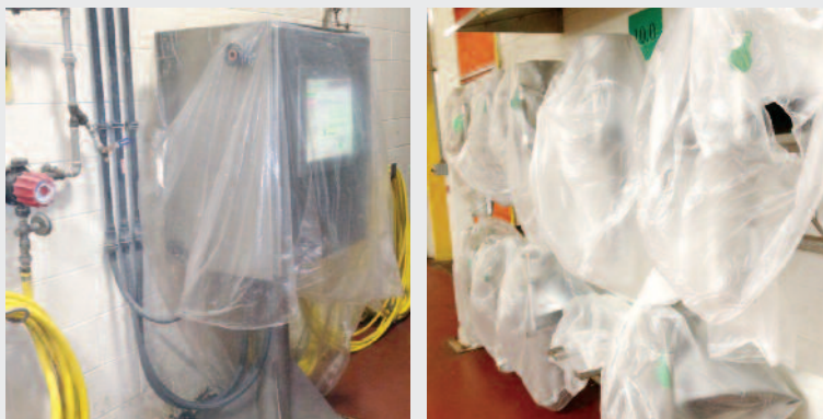
BEFORE: "Wash Down Sanitary Conditions" using disposable plastic, with open gaps and difficulty with installation.
