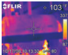
(After) Blanketed Y Strainer "Thermal Imaging Photography"
