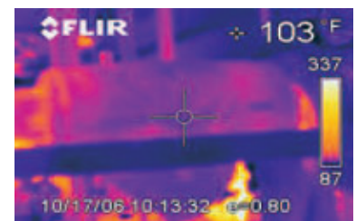
(After) Blanketed Y Strainer "Thermal Imaging Photography"
