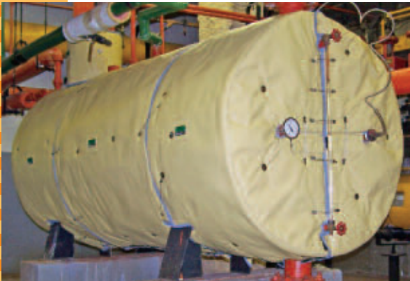
BUILDING MECHANICAL ROOM Steam Condensate Tank Design: LT450TT - 1.5" thickness Fastener: Stainless Steel Wiretwists
