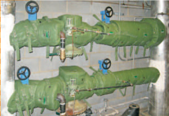
UNIV. CAMPUS – MECHANICAL ROOM Steam Reducing Stations Design: LT450TT - 1.5" thickness Fastener: "D" Ring Straps
