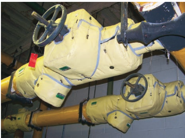
MAIN MECHANICAL ROOM – HP STEAM SUPPLY PRV STATION Design: LT450TT – “Yellow” PTFE Fabric Fastener: Stainless Steel Wiretwists and Velcro® Flaps
