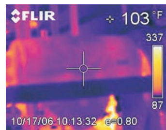
(After) Blanketed Y Strainer "Thermal Imaging Photography"
