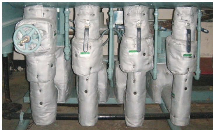
BOILER ROOM – FEED WATER PUMP, PIPING & VALVES Design: LT450SS - 1.5" thickness Fastener: Stainless Steel Wiretwists and Velcro® Flaps
