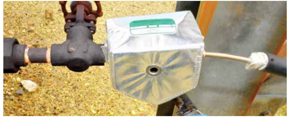
A Shannon Heat Shield, (Model LT500HS-AC) made with aluminized glass cloth, covering a thermostatic steam trap at a petroleum refinery. The Heat Shield includes a grommet for plant personnel to conduct ultrasonic testing on the trap via a probe along with Velcro fasteners to easily remove and reinstall the shield.
